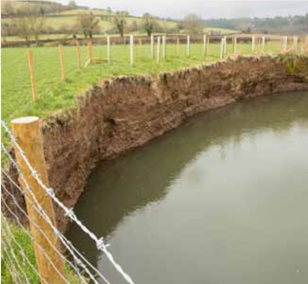
Bank erosion - the fence was placed two metres from the edge of the bank only one year ago
