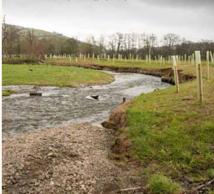
Bank revetment work, tree planting and willow faggoting all helping to stabilise the river bank
