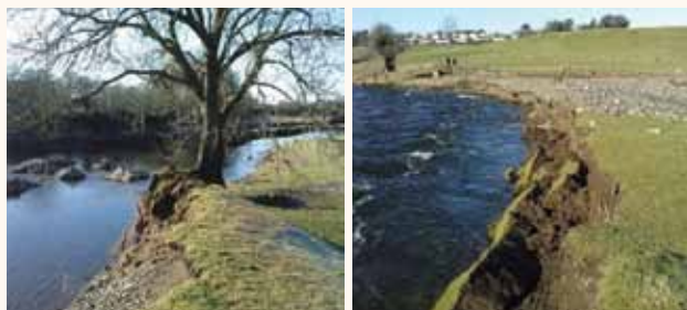
Examples of bank destabilisation on Paplava Farm at Cockermouth following flooding in 2009
